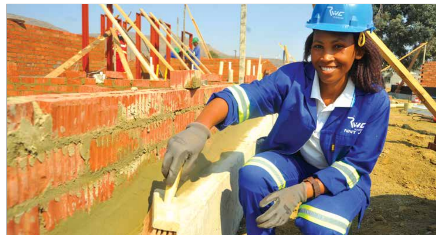
LOCAL LABOUR: Pictured is one of the workers on site Thandi Kahlulo (29) from Matatiele. Over 319 local jobs have been created at the Khotsong TB Hospital construction site in Matatiele.
