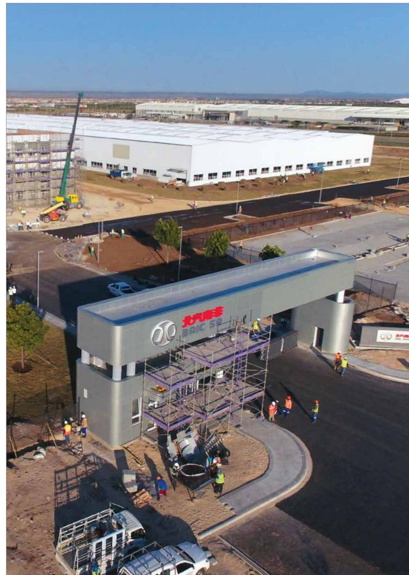
EMPOWERING GROWTH AND DEVELOPMENT: Progress is being made on the BAIC Group construction site, in Zone 1 of the Coega SEZ
